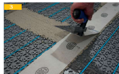
Corresponding system sealing elements (sealing tapes, sealing tape corners, sealing tape sleeves, etc.) are freshly embedded in the sealing adhesive and reworked.
